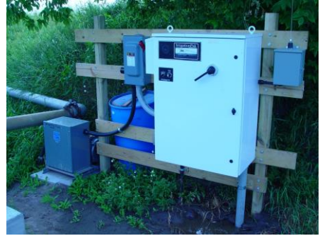
480V 1PH TO 3PH USING VFD
