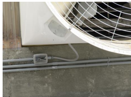
EACH FAN HAS ITS OWN O/C PROTECTION AND DISCONNECT
