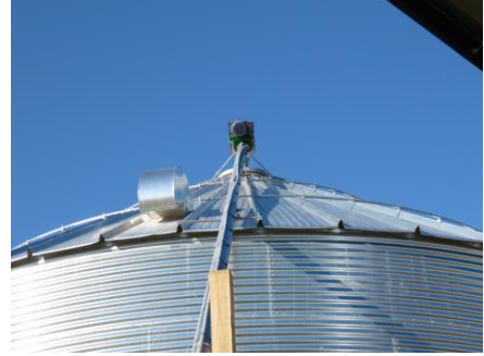
MOTORS ARE ALSO ON TOP. THEY DO REQUIRE A DISCONNECT WITHIN SITE
