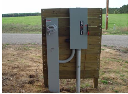
AT THE POINT OF SERVICE THE METER AND DISCONNECT
