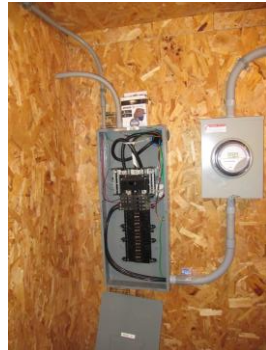
SECOND TOWER INPUT TO BREAKER
