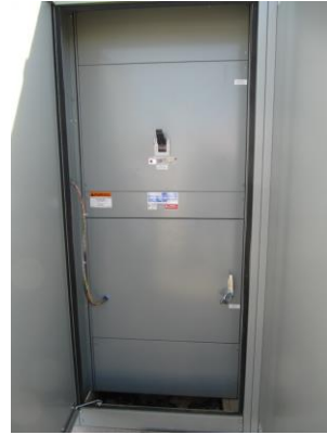
MAIN SERVICE DISCONNECT AND UTILITY CT SECTION
