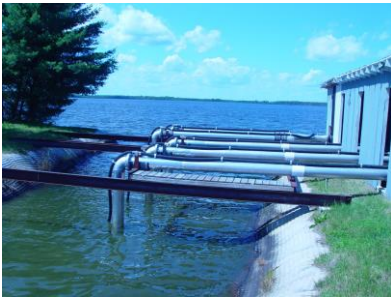
LARGE PUMPS PUMPING FROM LAKE
