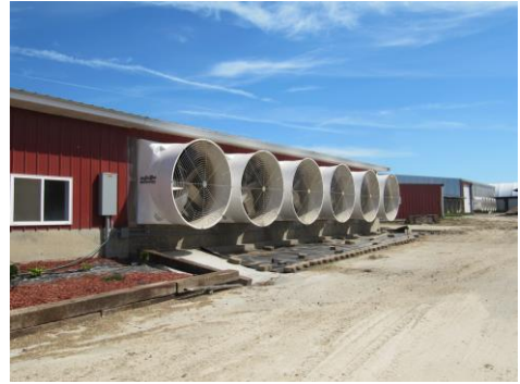
VENTILATION WIRING OFF SOLAR PWR
