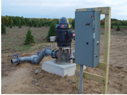
NEW WELL, PUMP AND 3PH PUMP PANEL
