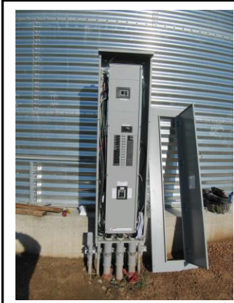
LARGE MULTI-BIN INSTALLATIONS TAKE A LOT OF POWER
