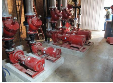
SEVERAL LARGE GAS BOILERS SERVE PROCESS
