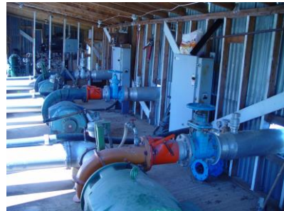
LARGE PUMPS PUMPING FROM LAKE
