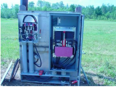
DRILLED WELL SERVICE SERVING PUMPS WHEN NEEDED
