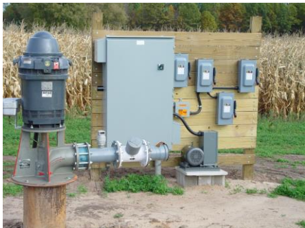
VFD DRIVE ALONG WITH ROTO PHASE FOR THE SMALLER 3PH LOADS
