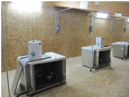
TYPICAL A/C UNITS ABOVE EACH SPACE
