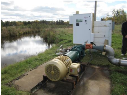
PUMP OUT OF LAKE NOT DRILLED WELL ALSO COMMON
