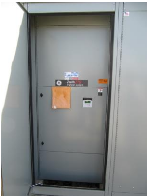
AUTOMATIC TRANSFER SWITCH SECTION
