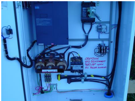
INTERIOR OF VFD
