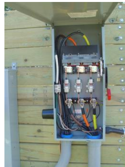
SERVICE RATED DISCONNECT ALSO SHOW LIGHTNING ARRESTOR
