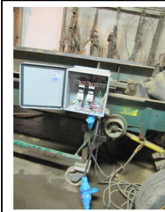
NEMA 4X BOX WITH CONTACTORS TO CONTROL OTHER EQUIPMENT
