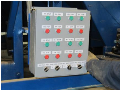
CONTROL PANEL FOR ALL THE VARIOUS CONVEYOR MOTORS
