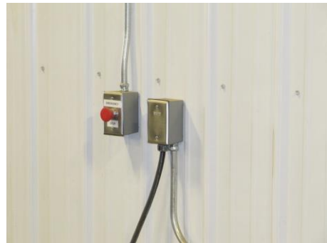
E-STOP AT EVERY WORK STATION
